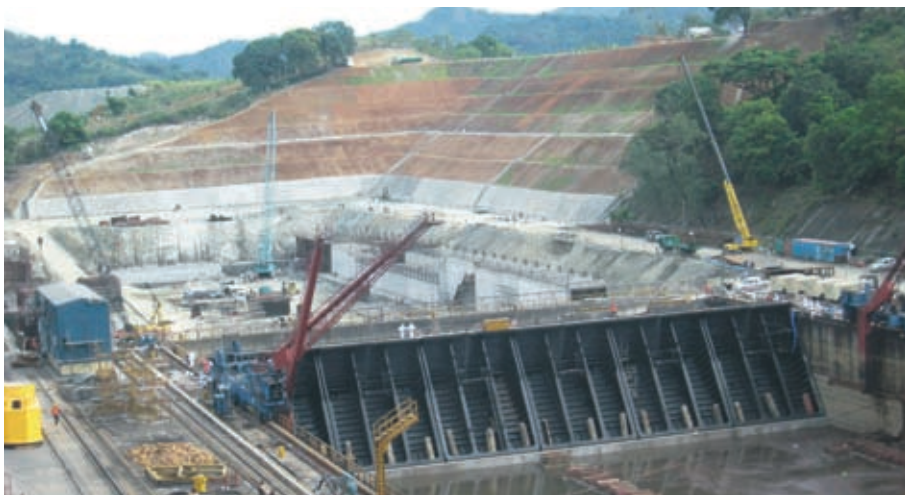
Civil works are ahead of schedule for the drydock expansion in Subic Shipyard
