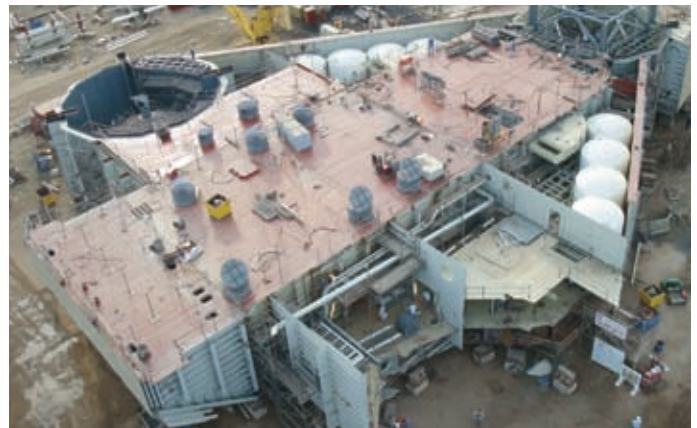
The hull of the first jackup taking shape on the shipyard's launchway
