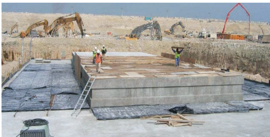
Construction of the yard in Qatar progressing well as workers prepare the floor slab panels in dock 2
