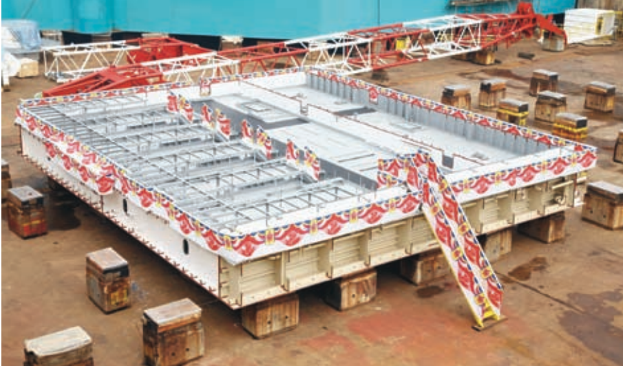
Keel of the fifth KFELS B Class jackup rig for SeaDrill was laid recently
