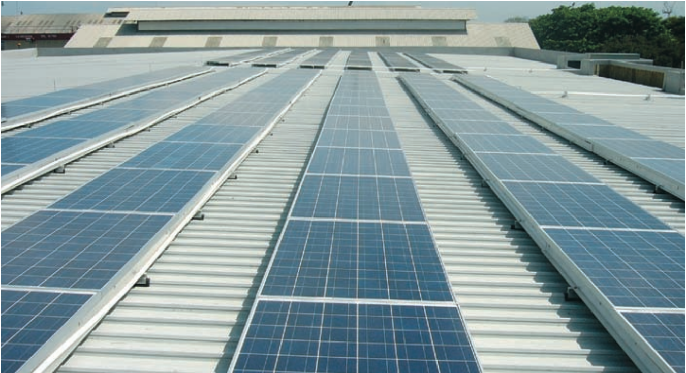
KOMtech has installed two PV cells power plants on its roof-top
