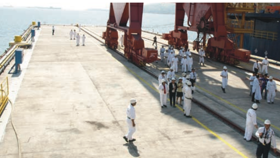
The newly extended Pacific Dock is able to accommodate the new generation of super large container vessels, VLCCs, containerships and bulk carriers
