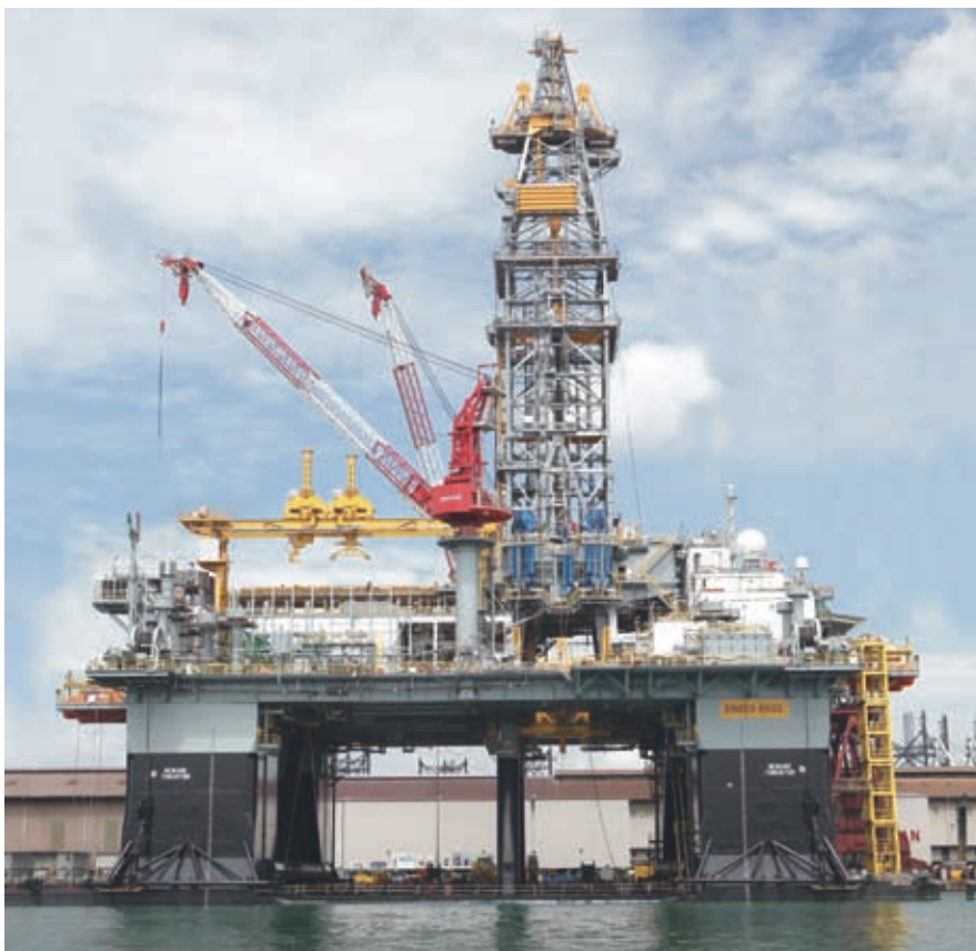
ENSCO 8502, the third of seven ENSCO 8500 Series® semisubmersibles that Keppel FELS has been contracted to build exclusively for EnSCO
