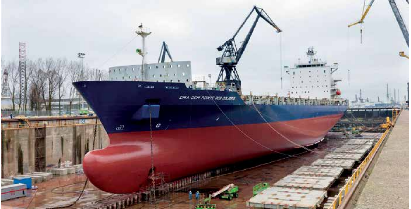
Having its repairs completed on time, within budget and safely, CMA CGM Ponte des Colibris (pictured), left Keppel Verolme's yard on 23 March 2016 and is scheduled for a long charter contract
