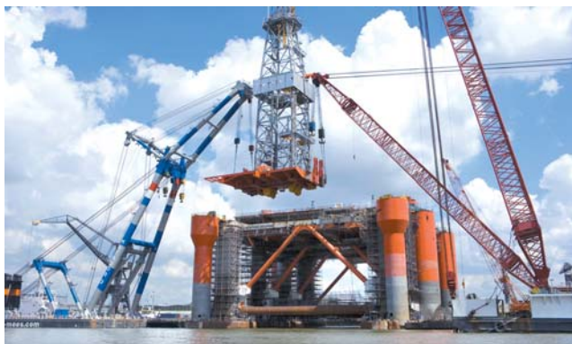
Keppel Verolme has completed the installation of the drill floor and derrick onboard Blackford Dolphin
