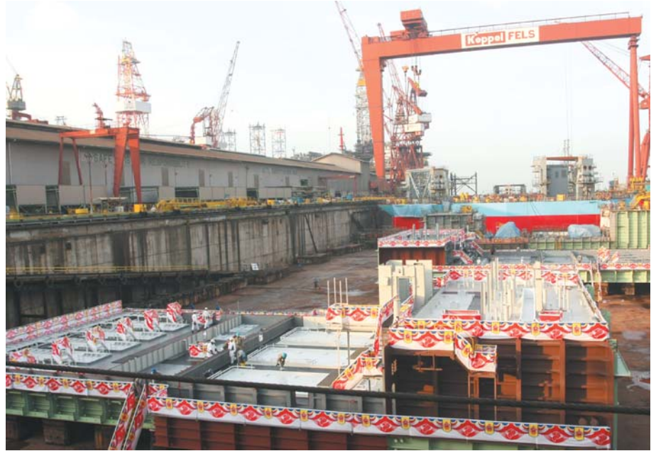
The first completed hull blocks of Deep Driller 8 and WilStrike are laid on keel blocks in the Admiral drydock
