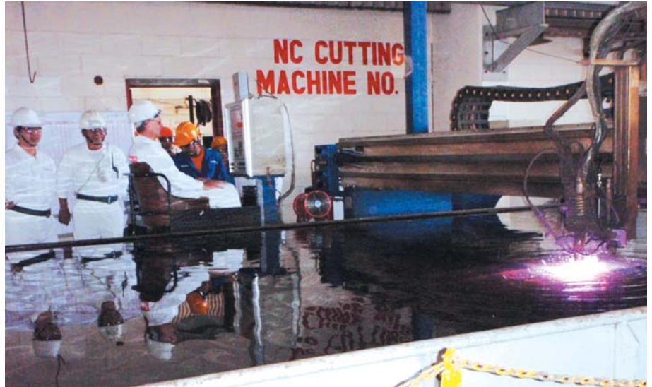
Strike steel marks the beginning of the physical construction work for each project
